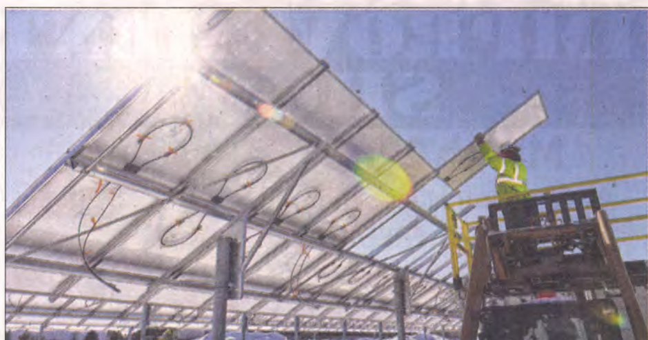
Chris Scheer, an electrician for Ranck Electric, helps guide into place one of the 3,000 solar panels that are going up in Lyon Township along I-96 near Old Plank Road. Each panel should be able to generate, at peak-wattage, about 700 watts of electricity. PHOTOS BY JOHN HEIDER | STAFF PHOTOGRAPHER
