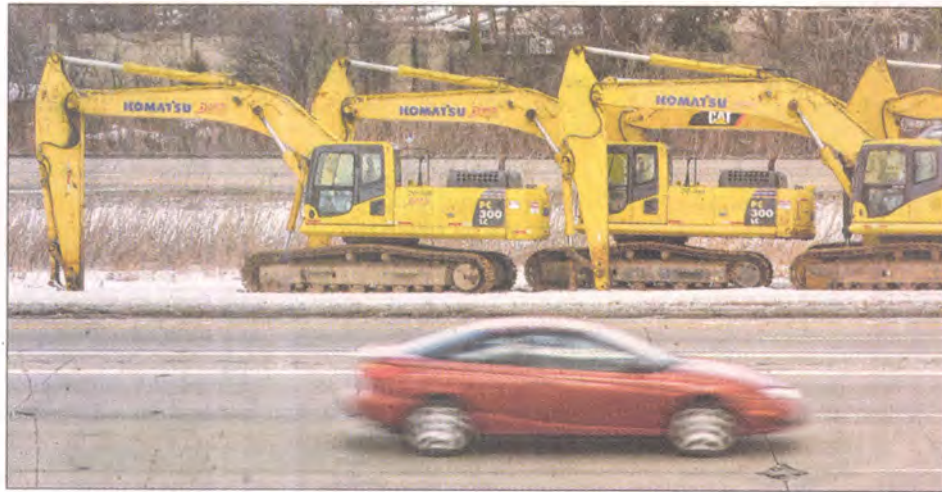
Construction equipment is staged on the I-96 median between I-275 and Newburgh Road. BILL BRESLER | STAFF PHOTOGRAPHER
