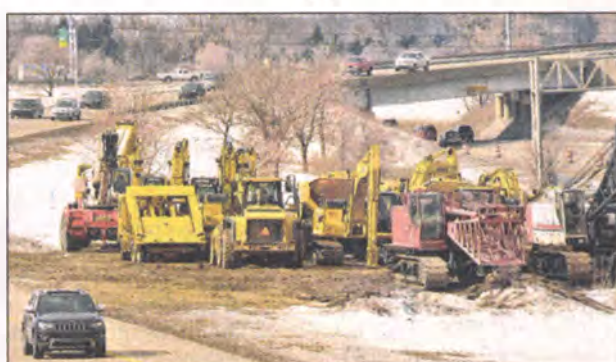
Construction equipment is staged on the I-96 median between I-275 and Newburgh Road. PHOTOS BY BILL BRESLER | STAFF PHOTOGRAPHER
