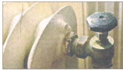
The original radiators are retained, but the entire heating plant was repaired and upgraded.
