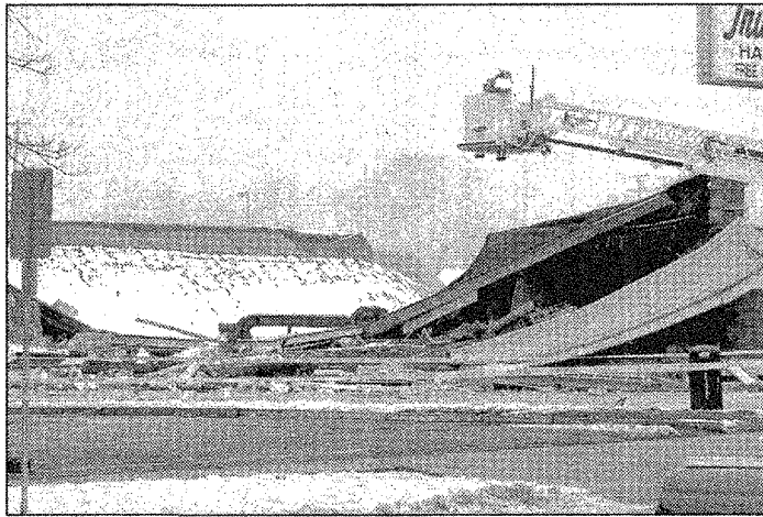
The roof of the furniture store fell to the ground in the explosion.
