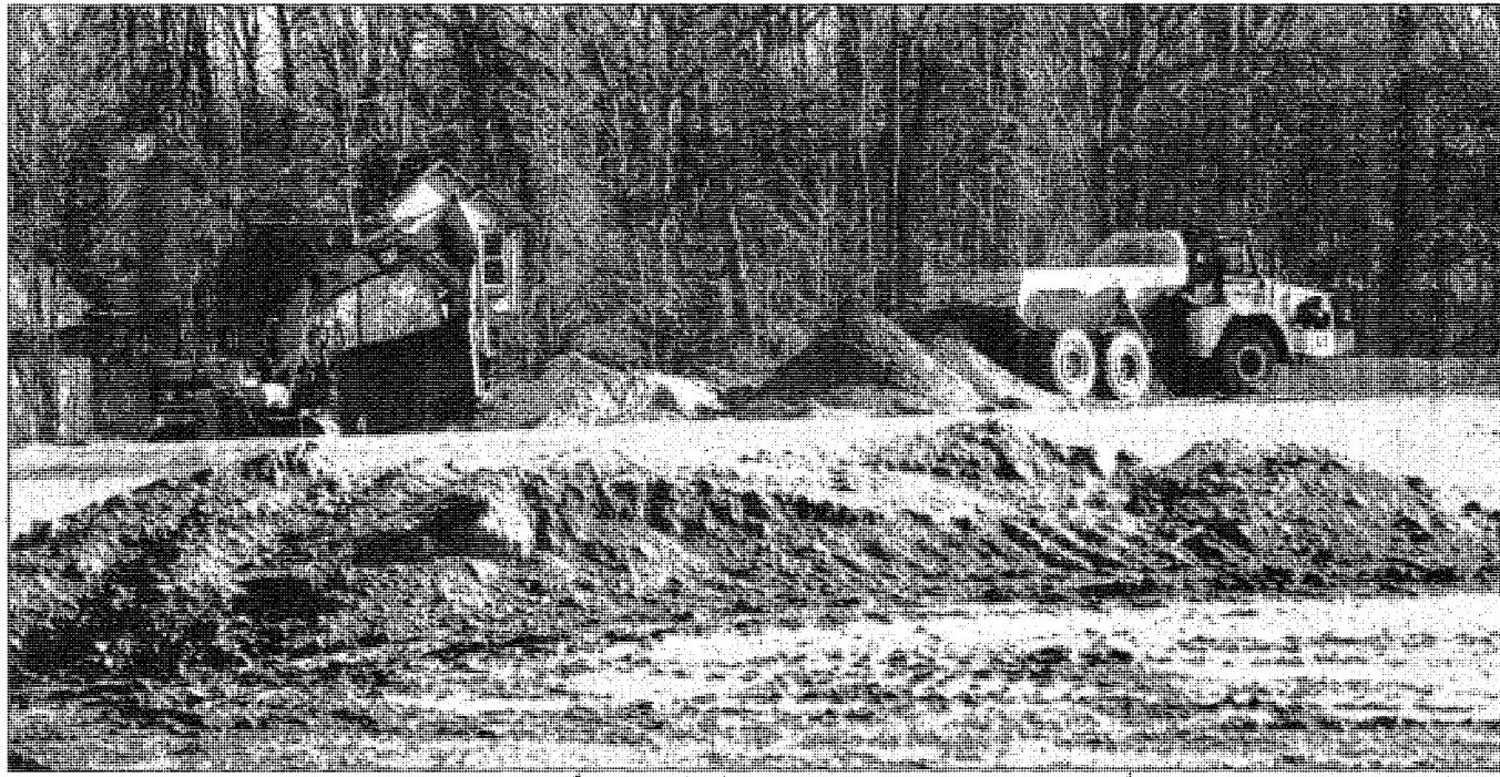
Soil is being moved as part of the Central City Park remediation and restoration. Work is expected to continue for a couple more weeks before ending for the winter.
