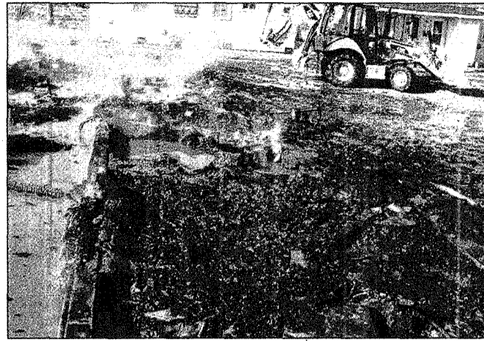
Charred debris and the foundation was all that was left of a four-unit apartment building on Manistee Court after an early morning blaze Wednesday.
