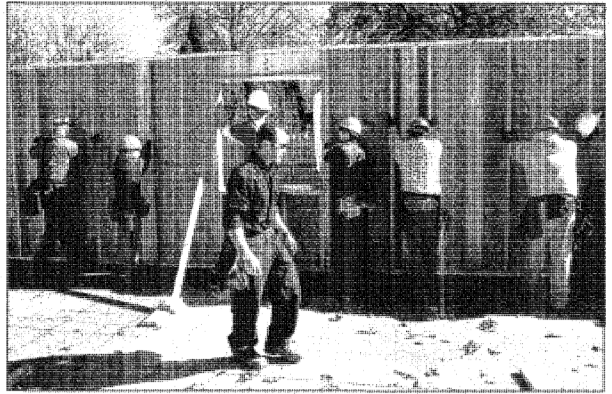
Construction Technology instructor Mark Valchine watches students working on raising walls on the home that's being constructed as part of a partnership with the Wayne-Westland Community Schools and the City of Westland.
