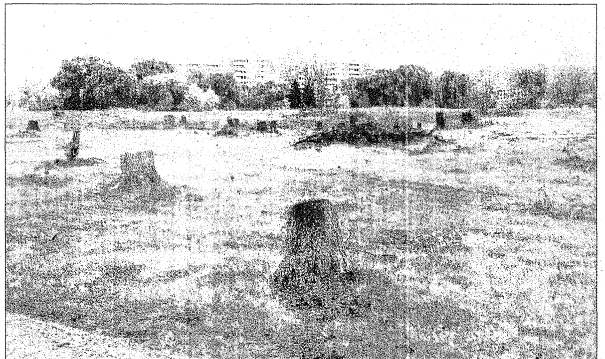
The stumps of trees mark the spot where work will begin on creating a new 12-acre Central City Park.
