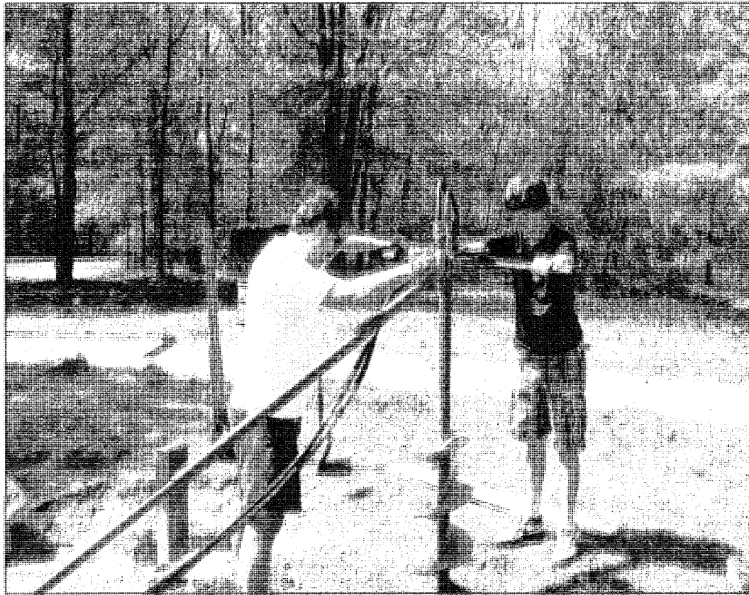
Cody Murphy and his father Jerry use a gas-powered auger to drill holes to cement in the posts for benches erected at the library pavilion.
