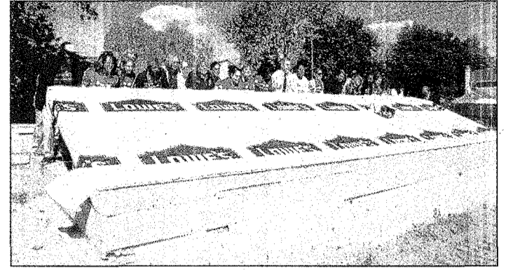
Volunteers including Westland Mayor William Wild lift the first wall at new construction home being built by Habitat for Humanity of Western Wayne home on Donnelly.
