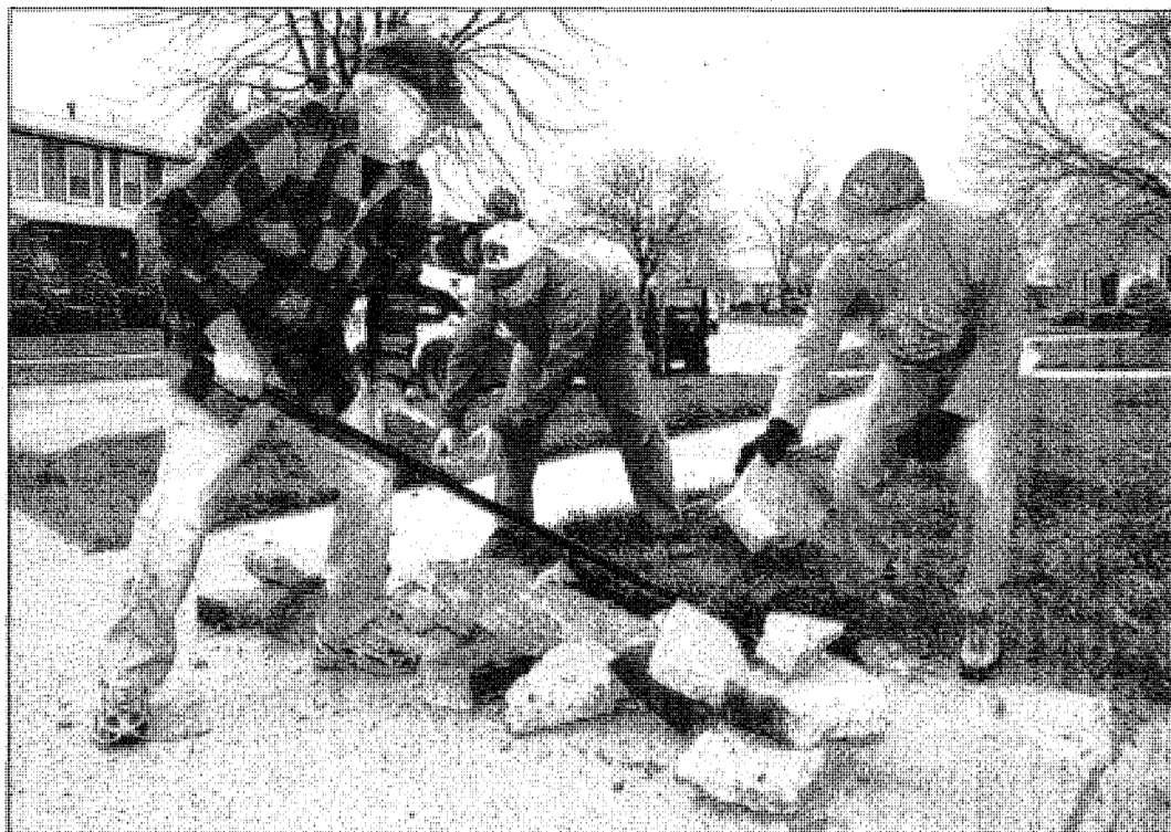
Keith Cox, Michael O'Hara and John Lutz break up a concrete driveway at Mary Stretke's house.
