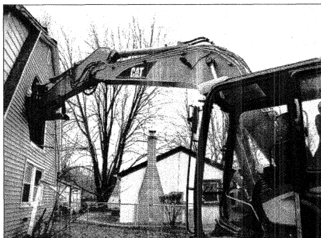
Westland Mayor William Wild takes a turn operating the excavator to begin the demolition of a dilapidated vacant home on Casco Court. It was the first home in Norwayne to be acquired and demolished through the federal Neighborhood Stabilization Program.
