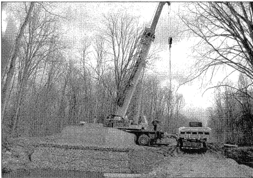
Work crews haul one of the bridges into the recreation area and prepare to place it over the Lower Rouge River.
