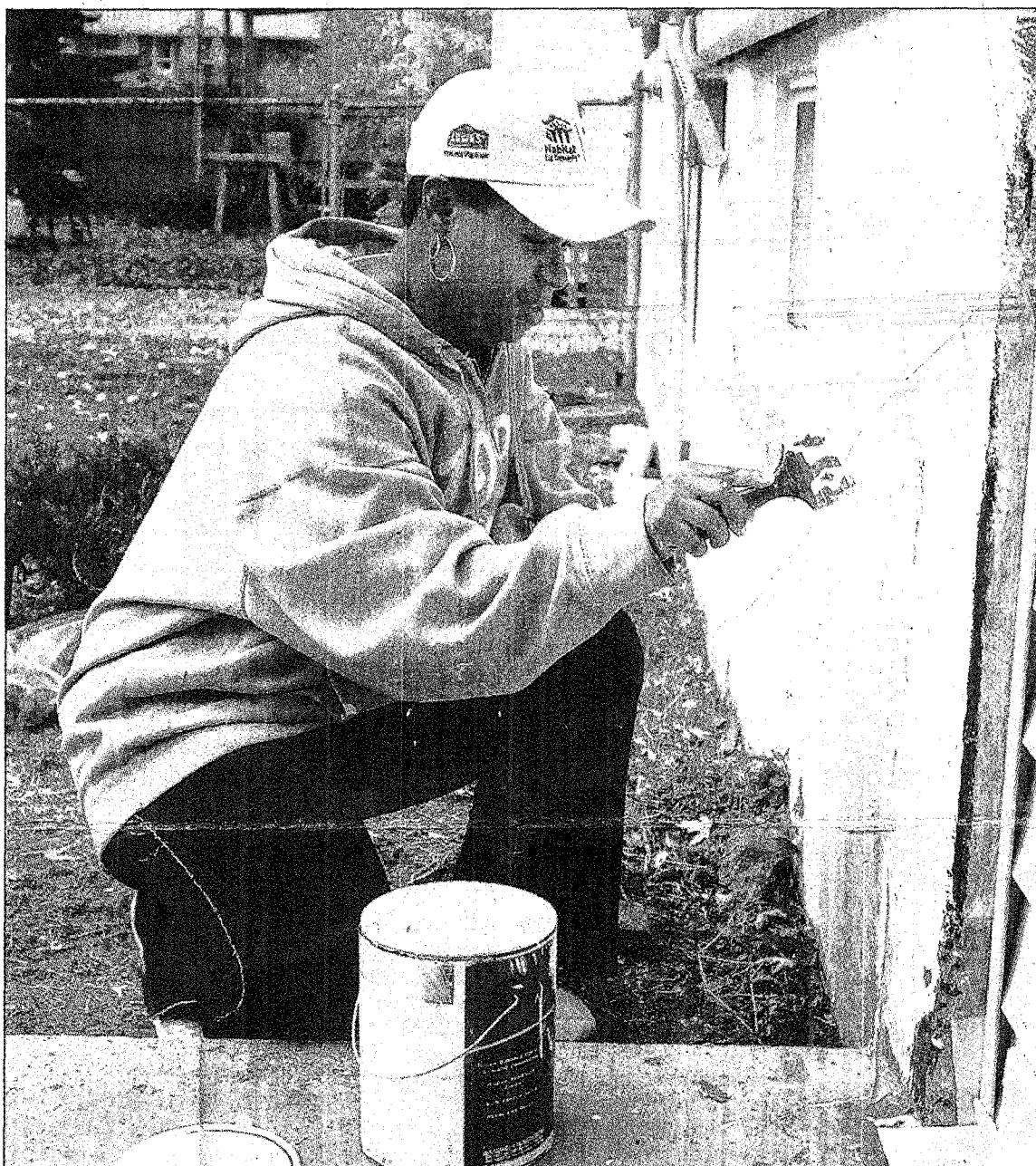
Kenette Washington does exterior painting as part of the 750 hours of sweat equity she is doing to get her Habitat for Humanity home in Westland.
