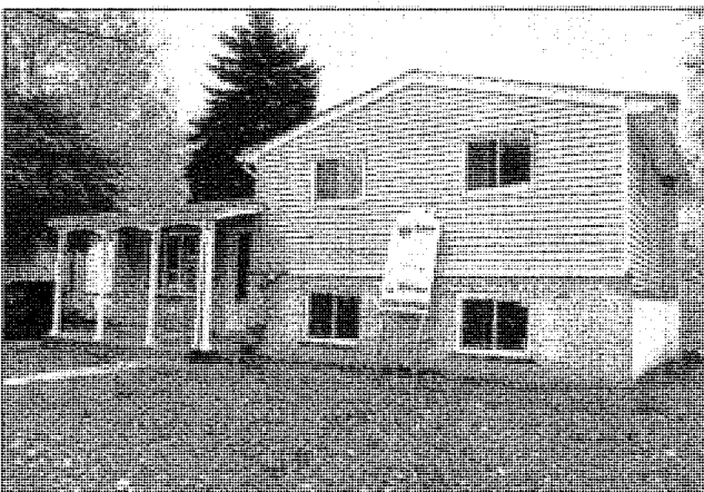
A tri-level home on Vincent Street is being rehabilitated by Habitat for Humanity of Western Wayne in partnership with the City of Westland.
