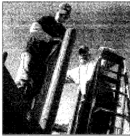
Michael Yates of GameTime (left) and volunteer Bernie Brewer of the Wayne Masonic Lodge #12 in Westland place a panel on the new play structure.
