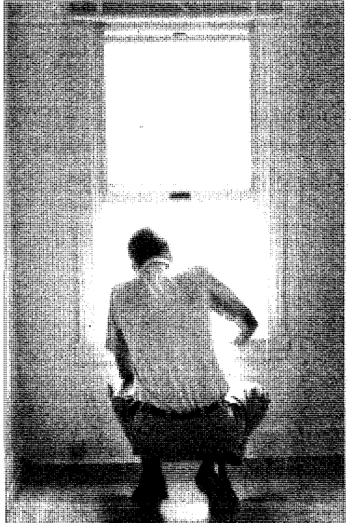
Bill Tremper watches carpenter Ron Bruce work on the porch from the widow of one of two rooms upstairs yet to be renovated.
