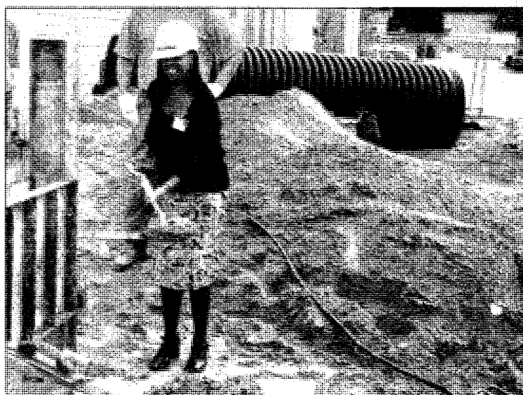
Shelly Clark, Garden City Hospital's manager of patient registration, pours the first shovelful of concrete for the new surgical center.
