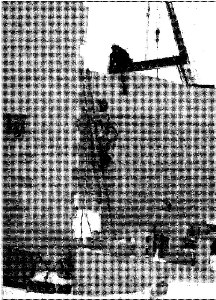
Work began last fall on Schoolcraft's new Biomedical Technology Center. Construction crews are now putting walls in place. The $12.5 million building is scheduled to open in fall 2008.
