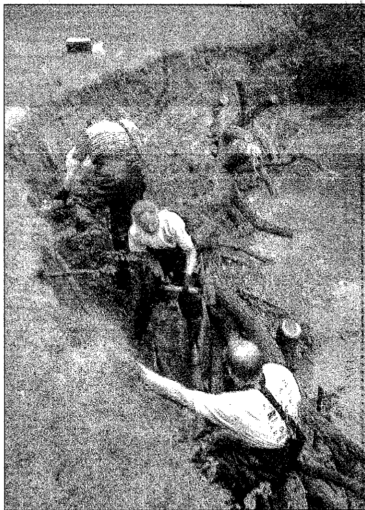
Friends of the Rouge have been instrumental in a number of streambank stabilization projects, including this effort on a Rouge tributary in Birmingham last year.
