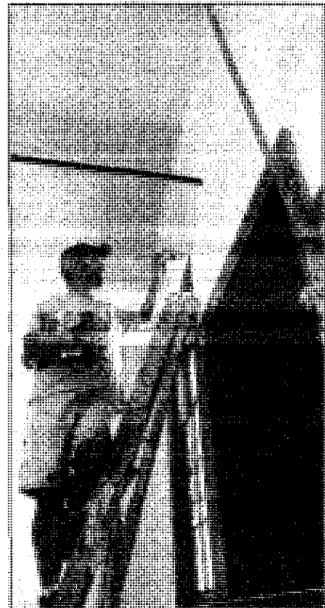
Painter Gary Martin touches up around one of the windows in the school.
